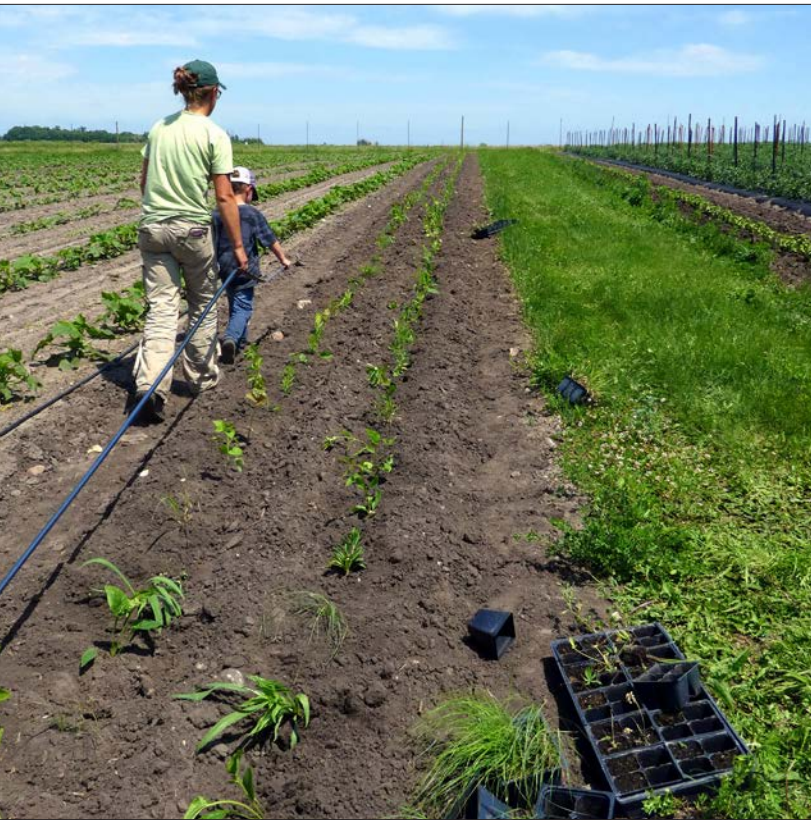
Figure 4.14: Installing drip-tube irrigation to help establish plant plugs in a Minnesota pollinator planting.
