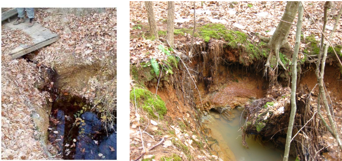
Figure 12: Examples of Headcuts (NC DWQ, 2004)
